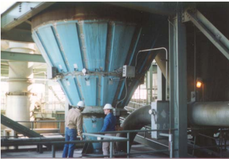
← COAL SILO HEATED WITH FRP HEATING PANELS AT A MAJOR UTILITY IN THE NORTH EAST, USA
