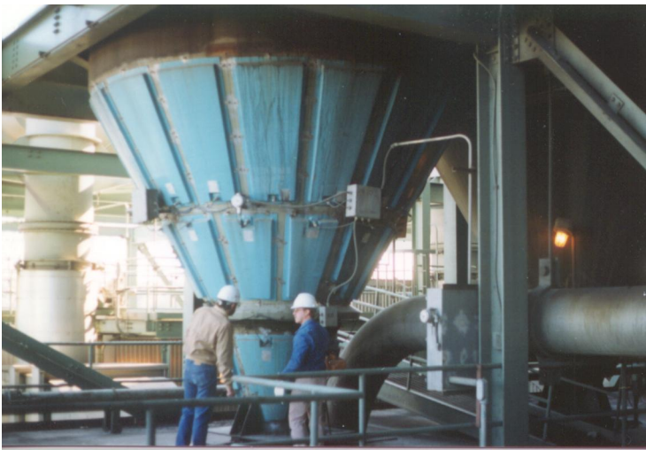
← COAL SILO HEATED WITH FRP HEATING PANELS AT A MAJOR UTILITY IN THE NORTH EAST, USA
