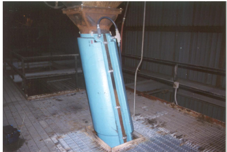
▶ SAMPLING CHUTE, 12" DIAMETER, HEATED WITH FRP HEATING PANELS
